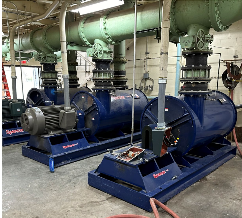
Existing Centrifugal Aeration Blowers
