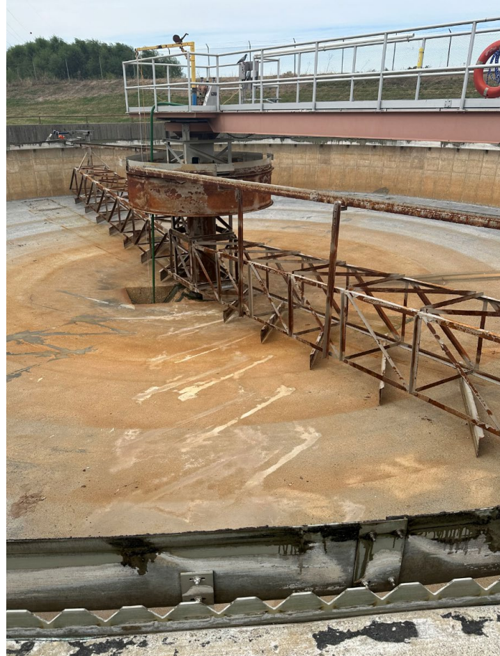
Primary Clarifier Equipment, Weirs and Baffles
