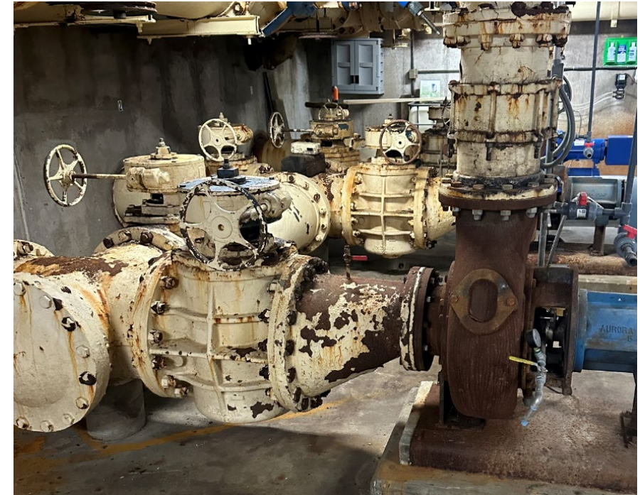
RAS Sludge Pumps and Piping
