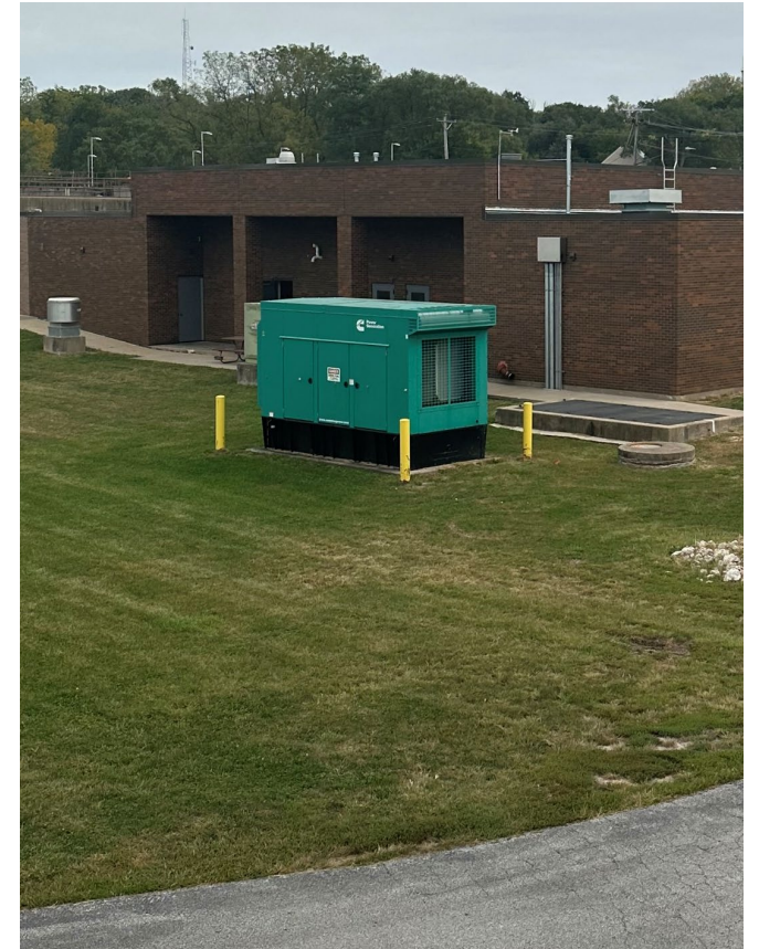
Backup Generators, Electrical & SCADA
