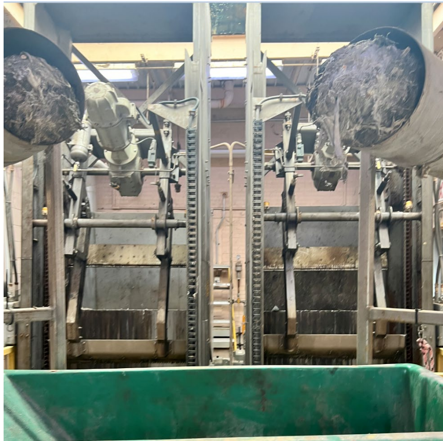
Influent Screening Room
