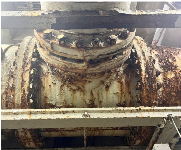
Influent Pump Station
