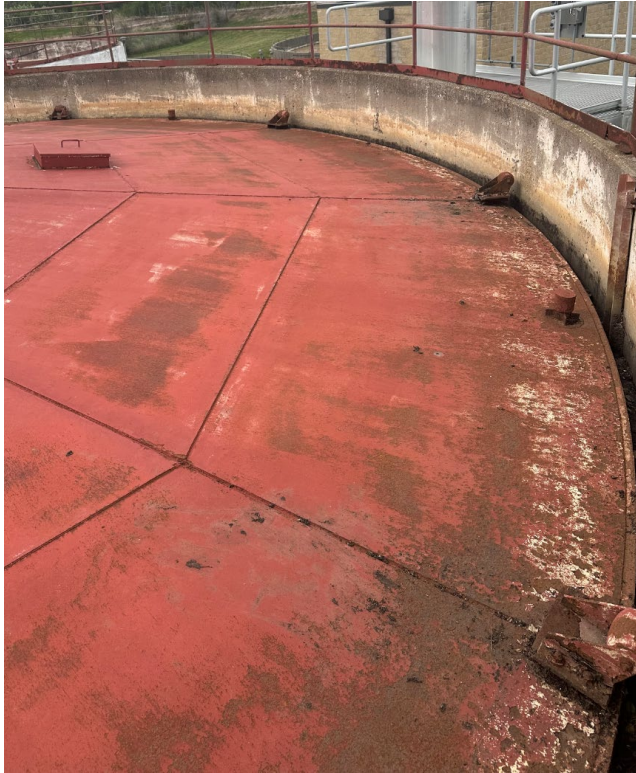
Anaerobic Digester Covers
