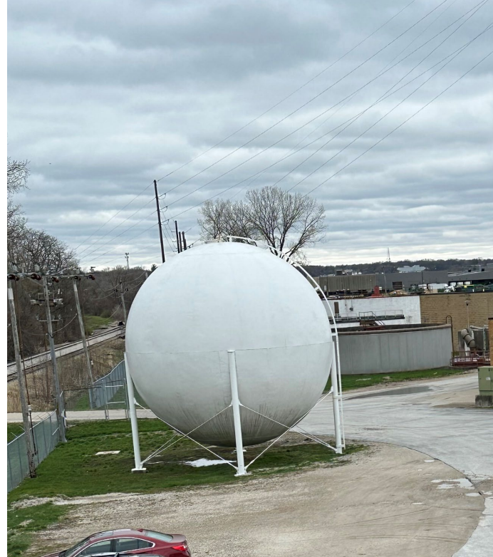
Biogas Holding Sphere
