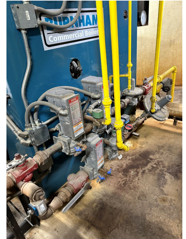
Boilers for Anaerobic Digesters (biogas is currently flared)
